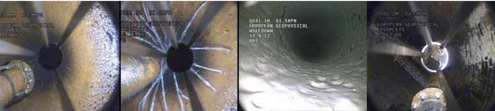
Rising main join in 600mm plain steel lined borehole
